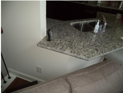
GFCI protection needed at the outlet below the kitchen counter given the proximity to the kitchen counter/ sink area.
