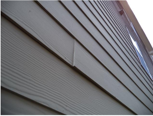
Loose cement composite siding noted at the left side of the home near the electrical meter.
