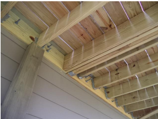
Band joists lack end bearing at the interior run at the added deck area.
