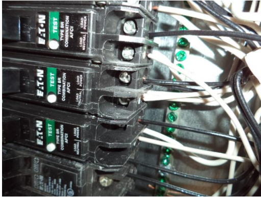
Double taps noted at AFCI breaker for slot #19.
