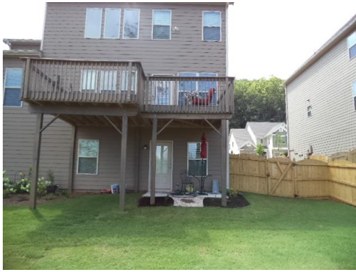
Decks(s) show indications of settlement or lack of construction in plumb.
