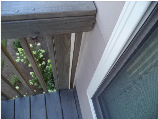
Loose railing and baluster noted at the added deck area.
