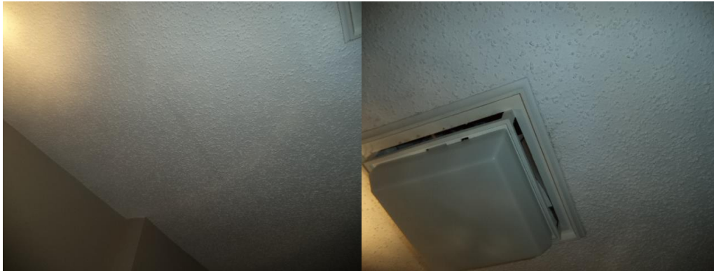
Localized water staining noted at the master bathroom area.
