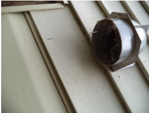
Recommend installing a proper dryer vent cover at the front left corner of the home.
