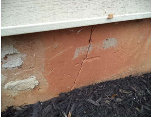
Settlement cracking noted at the front wall.
