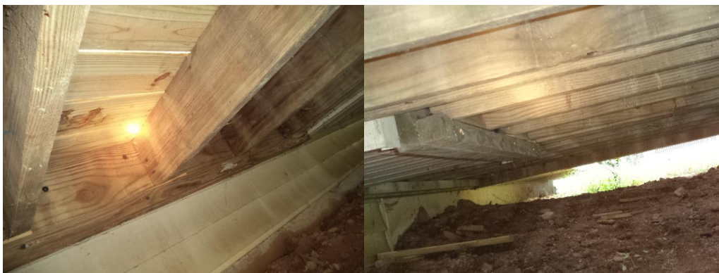
Deck lacks flashing with proper anchorage/ lagging with failing end bearing for joists at interior ledgers.
