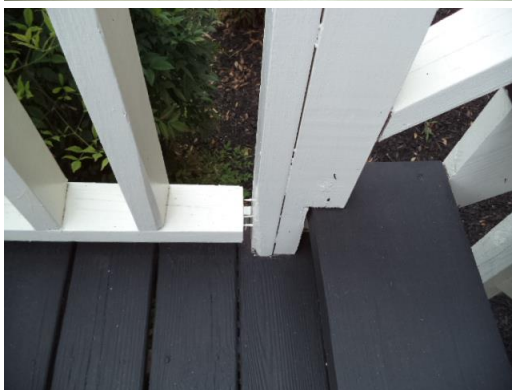
Front porch lacks lagging/ anchorage with loose railings and excessive openings.
