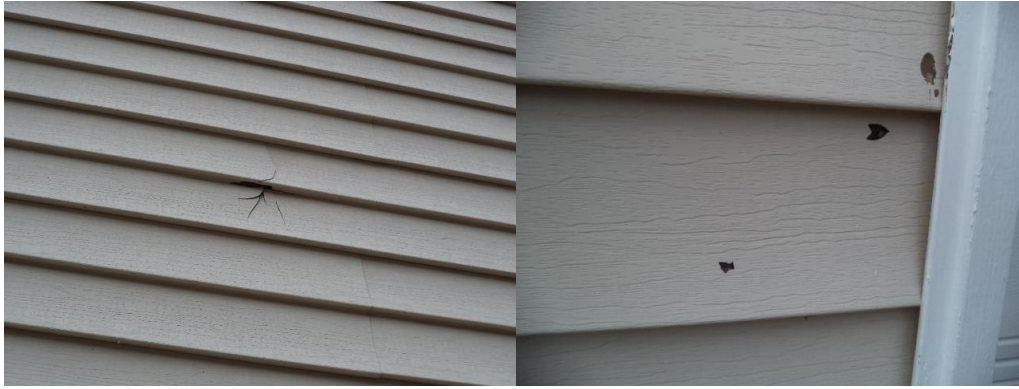
Localized damage noted in the vinyl siding.
