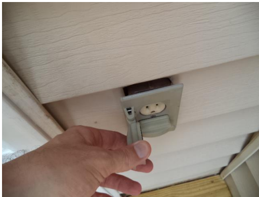
Loose outlet noted at the rear exterior.
