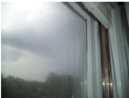
Lost seal noted in the 2 nd floor hall bathroom window.
