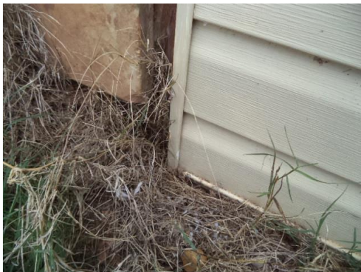
Siding to grade proximity issues noted at the front and left sides of the home.
