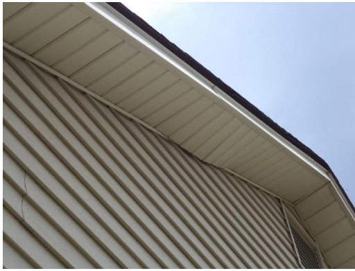
Loose soffits noted at the left side of the home.
