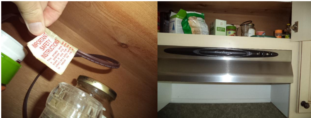
Extension/ appliance cord splicing noted at the kitchen vent unit.
