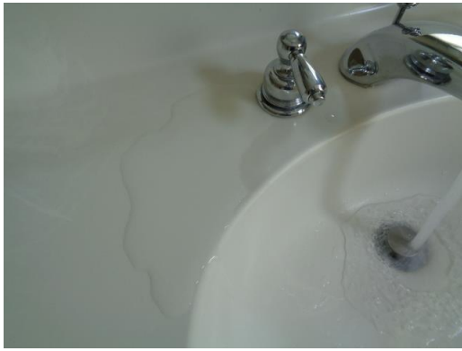
Leaky fixtures noted at the master bathroom sink hot sides.
