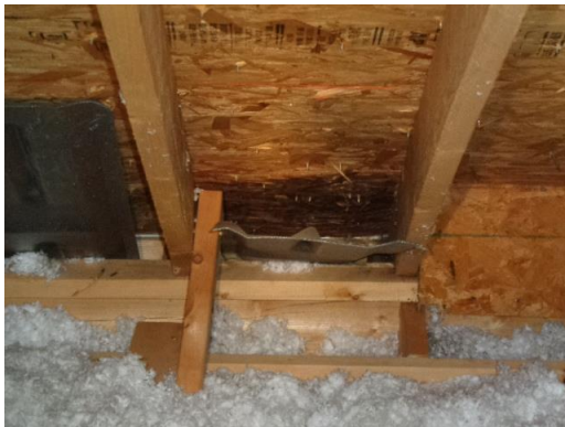
Evidence of roof leakage near the chimney chase.
