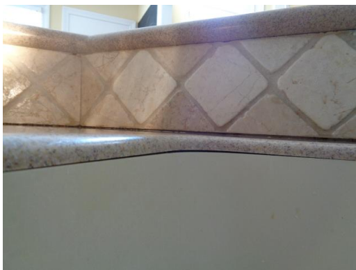
The inset sink fixture is separating from the countertop at the kitchen.
