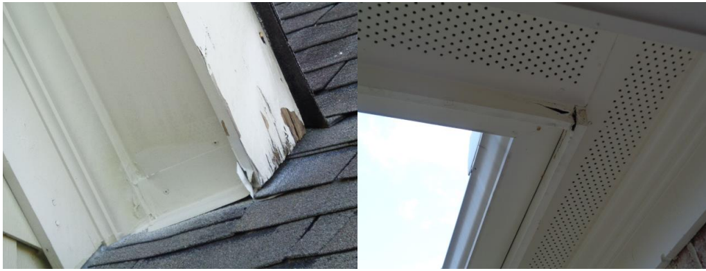
Localized rot noted in the fascia at the front of the home.
