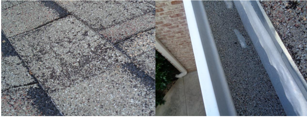
Atlas chalet shingle material noted at the home with excessive granule loss noted in areas.
