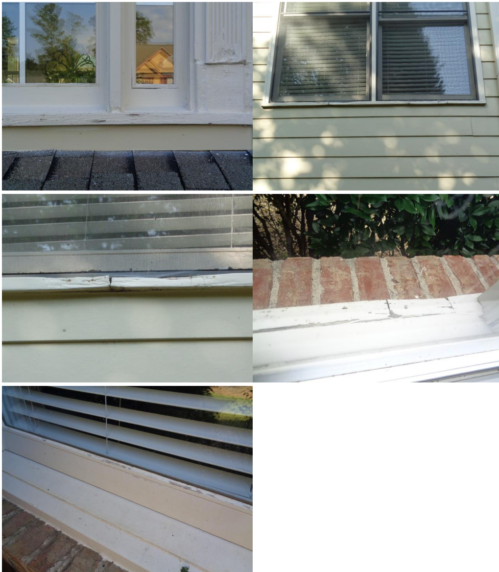
Localized rot noted in windows at the front and rear of the home with painting needed.
