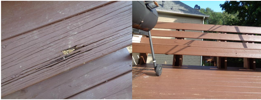
Loose/ damaged treads noted at the deck stairs and excessive openings noted at the deck bench areas.
