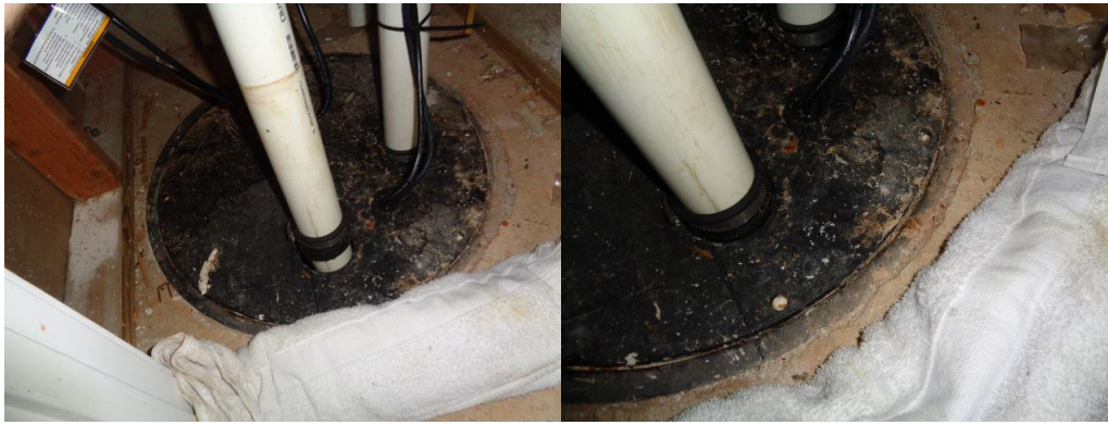
Evidence of amateur sump pump installation at the basement with venting and leakage issues noted.
