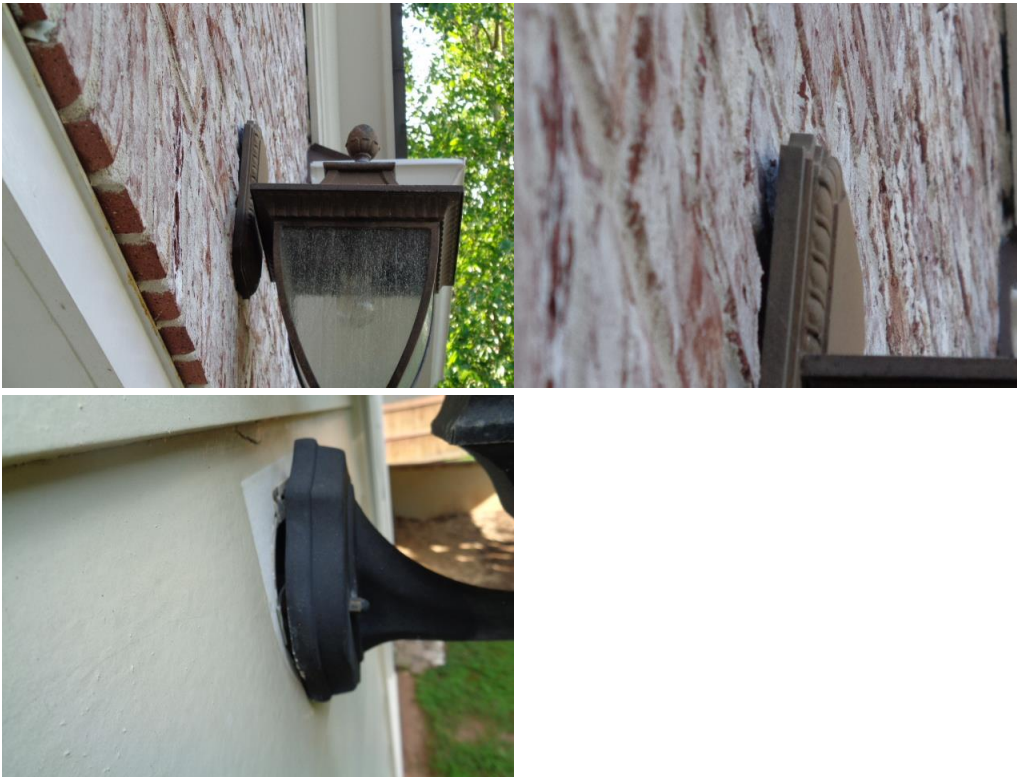
Recommend securing and sealing exterior light fixtures.
