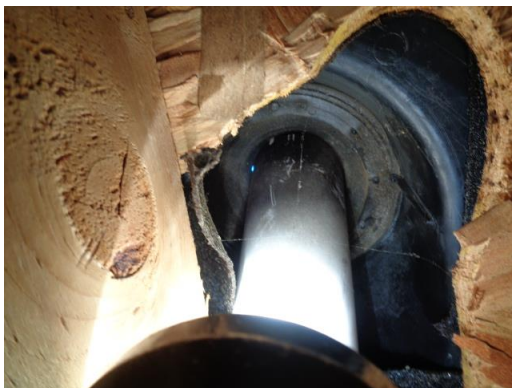
Light showing around neoprene boot flashings.
