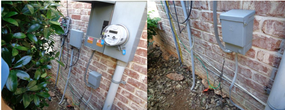
Exposed wiring and no over current protection noted at the meter and heat pump unit.
