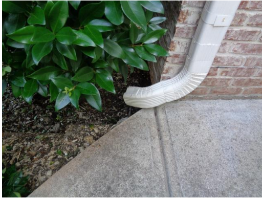
Recommend extending downspouts away from the vulnerable area at the front entry.
