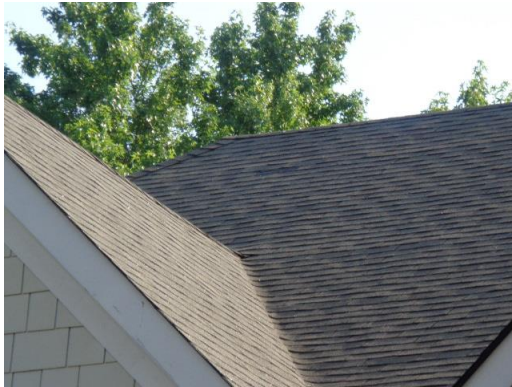
Missing roofing material noted at the front slope.
