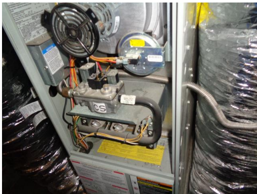
Gas supply improperly flex piped into the furnace burner compartments.
