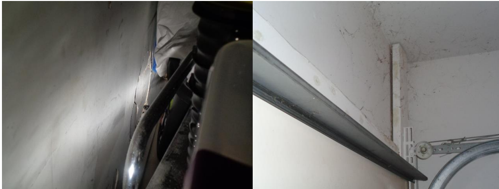
Firewall damage and loose mounting ledgers noted at the garage area.
