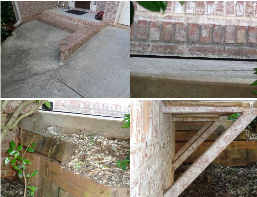
Settlement and backfill issues with movement in the retaining wall noted at the front entry.
