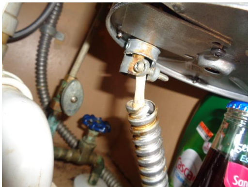
Loose/ damaged conduit noted at the waste disposal circuit.
