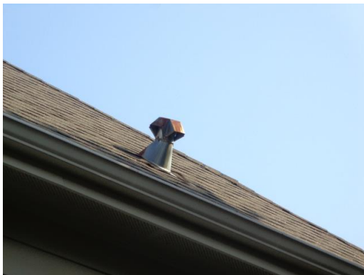
Rusting noted in the exhaust vent cover at the right side roof slope.
