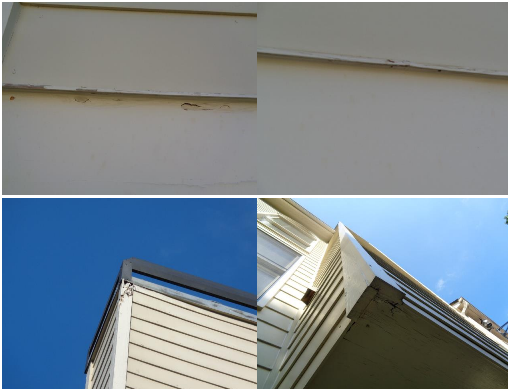
Rot noted at the chimney chase area and wood trim at the sides of the home between the claddings.
